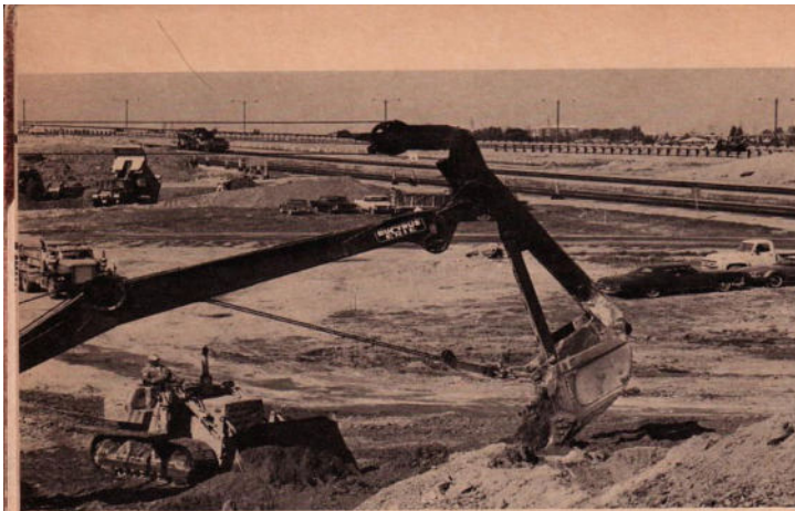
HIGHWAY widening is well under way when storm sewer trench is backfilled.
