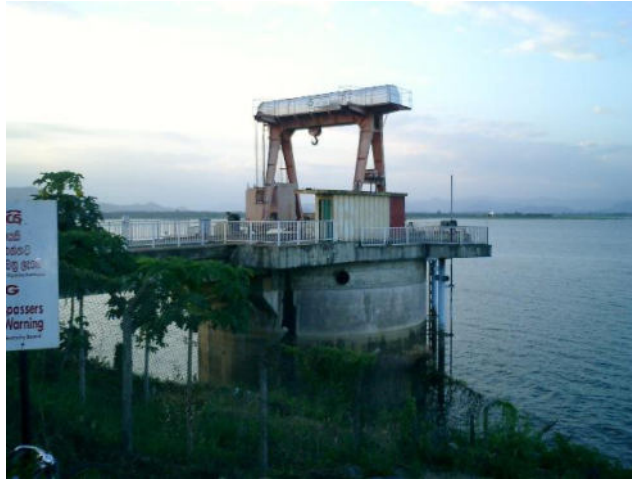
RIGHT BANK POWER PLANT AT UDAWALAWE PROJECT. PICTURE TAKEN IN JANUARY 2005
