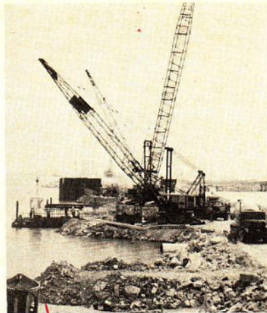
VIEW is south from shore. Footings for pier are placed from causeway.
