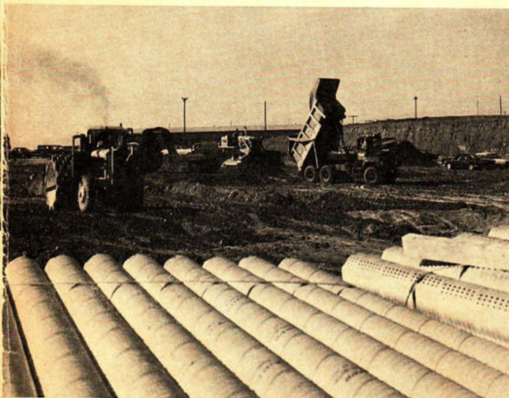
GRADING for project on Macdonald-Cartier freeway involves 1,300,000 cu yd of material; 900,000 cu yd was brought in; 200,000 cu yd excavated on site.
