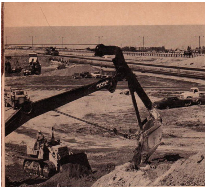
HIGHWAY widening is well under way when storm sewer trench is backfilled.
